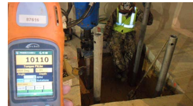
Installing four helicals to support dual beams. Pro-Dig handheld display assisting with the installation to insure lasting stability of the helical designs.
