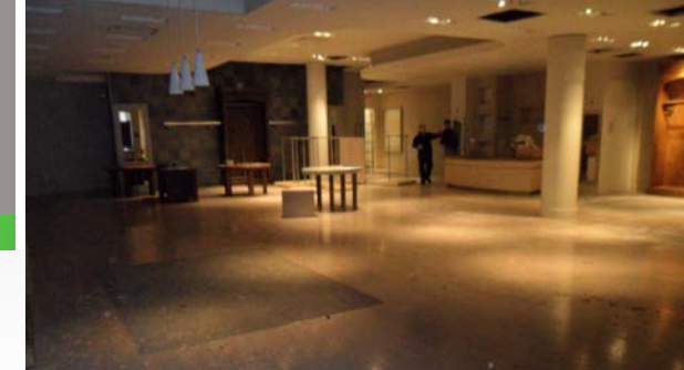
Visible columns before renovations. Columns will be removed and replaced with new beams around the perimeter to distribute the weight of the floor above.
